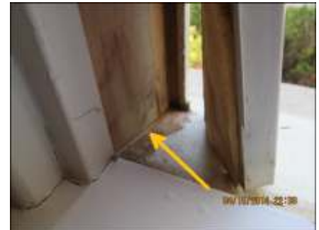
View behind UNSEALED window tracks. Moisture below.
