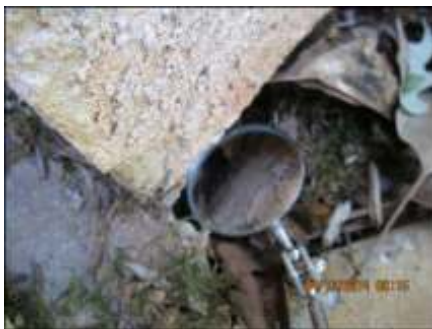
Mirror shows stucco foam is sealed at bottom
