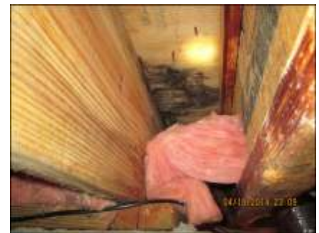
Attic view of moisture damage from improper kick-out flashing
