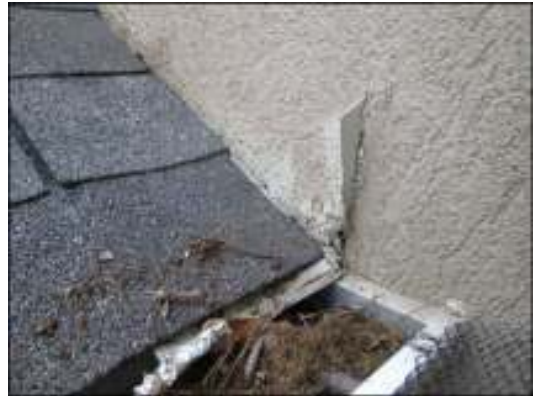
Photo B: Gutters need to be cleaned
