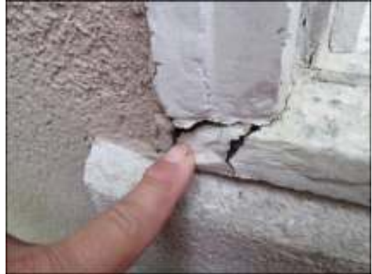
Photo 2: Sample photo of window sill rot at front left window. Recommend repair.
