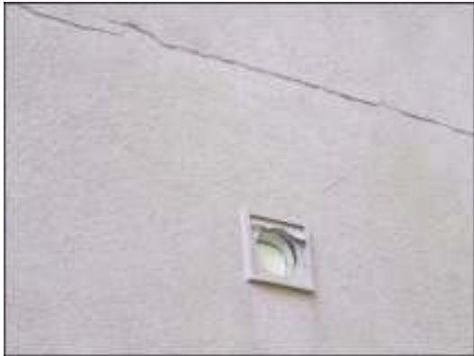
Photo A: Dryer vent is damaged. Recommend repair.
