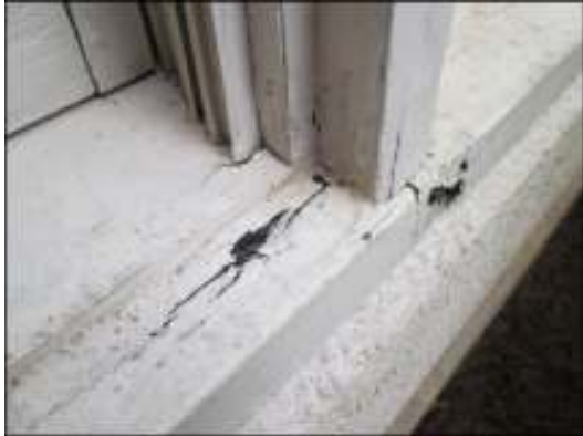
Photo 1: Sample photo of window sill wood rot. Needs repair
